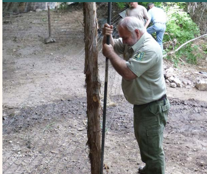
USFS member building fence for a protection barrier at Castle Springs. Credit: USFS
